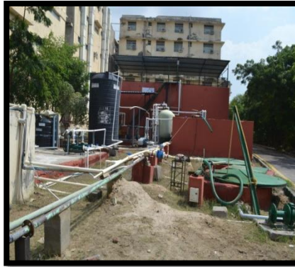
Sewage Treatment Plant (STP)
