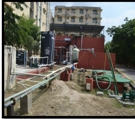
Sewage Treatment Plant (STP)
