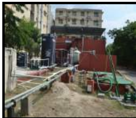
Sewage Treatment Plant (STP)
