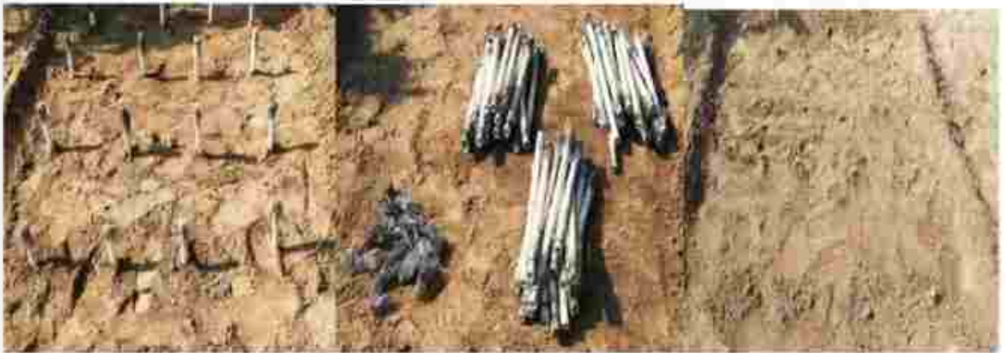
Earth Recharge Pipes
