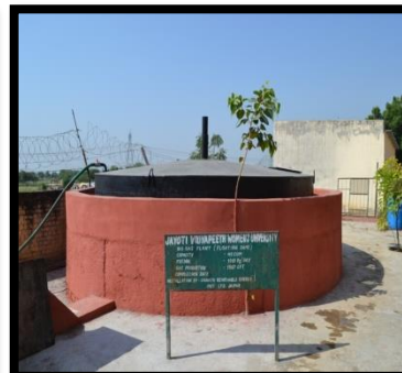
Figure 9 Bio Gas Plant
