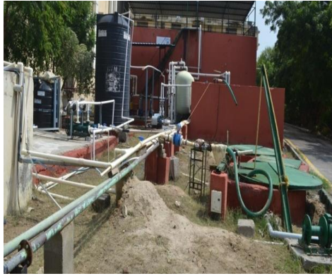
Figure 1 Sewage Treatment Plant (STP)
