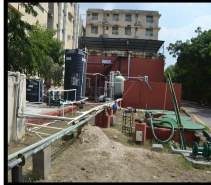
Figure 13 Sewage Treatment Plant (STP)
